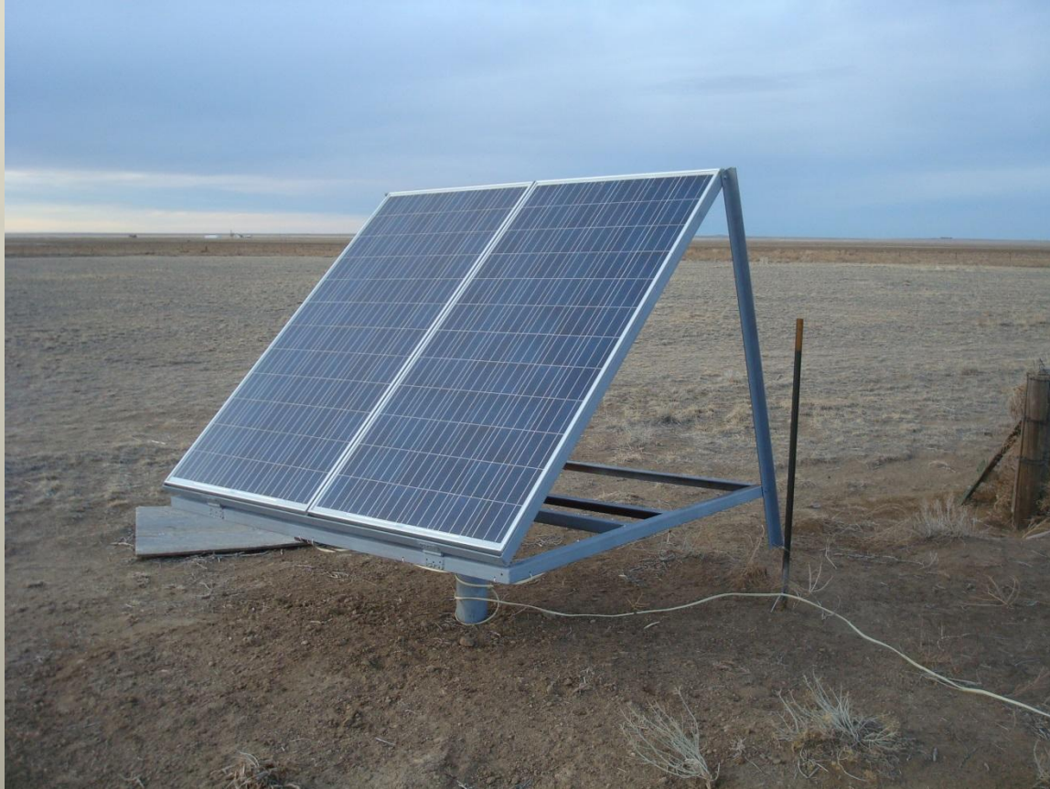
Solar panels for bunker batteries
